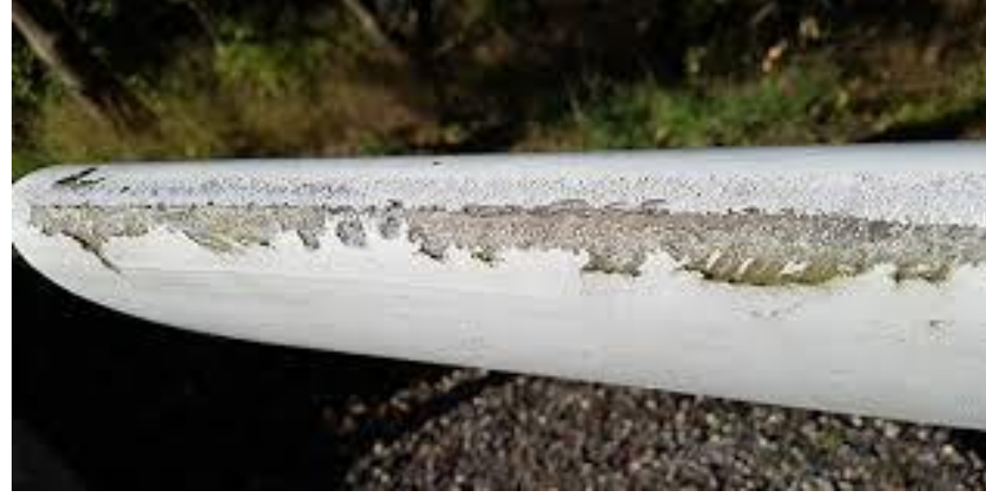
Wind turbine blade with damage on the leading edge Courtesy of Jakob Ilsted Beck
